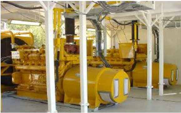
Figure 2. Engine Generator Sets
